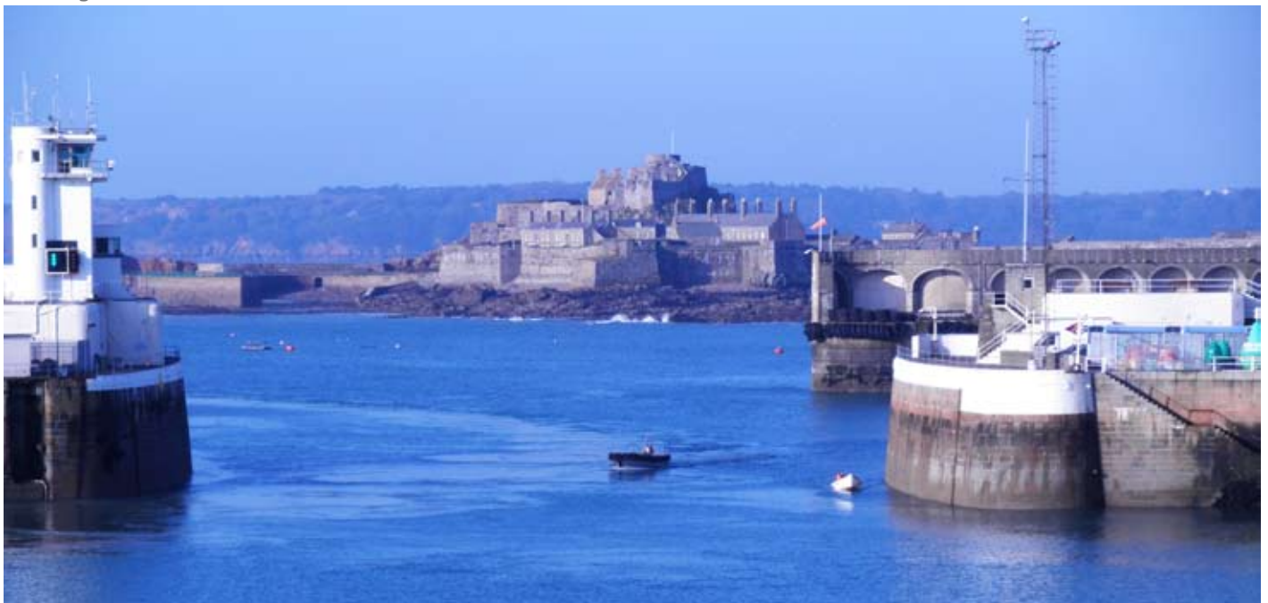
Rockbond Underwater Mortar use to protect concrete piers against scour attack at the Queen Elizabeth Ferry at Jersey Port, Channel Islands.
